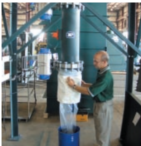
BIBO dust discharge. Hazardous compounds contained during BIBO filter change.
